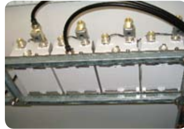
SASU to reuse existing 2G site antenna and feeder system
